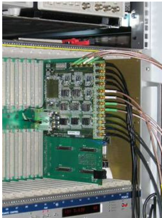
Figure JRA1.9.11: SIMCON3.0 ready for tests.
