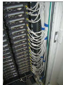
Figure 5: Cabling inside the rack
