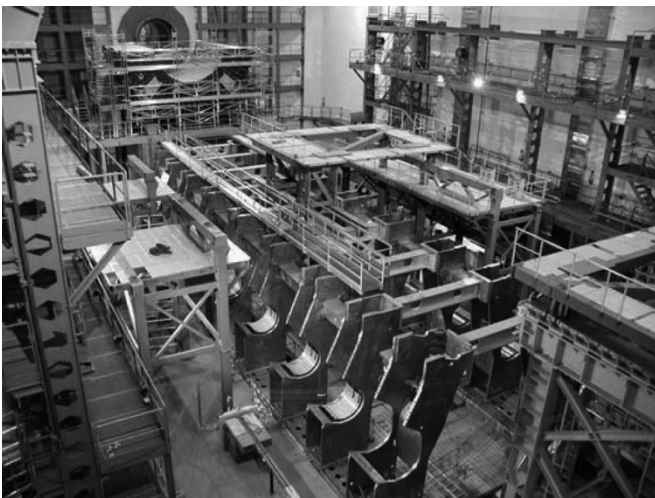
Fig. 9. ATLAS cavern 100 m underground, outer structures and feet installed, ready for receiving the Barrel Toroid coil in Oct 04.
