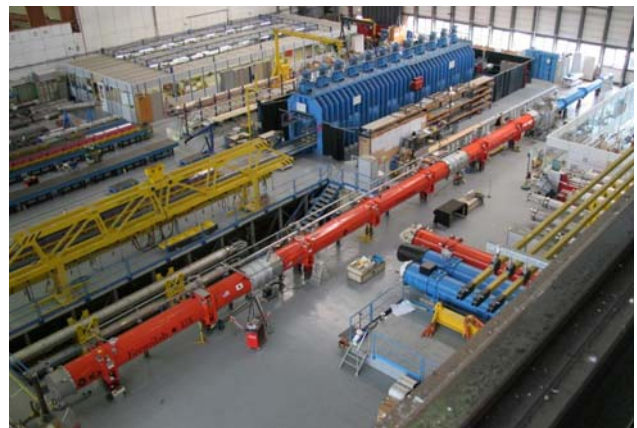
Figure 6. LHC Low- \beta triplet assembled at CERN before installation in the LHC tunnel.
