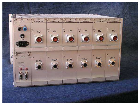
Figure 3. HCAL HPD power supply crate.
