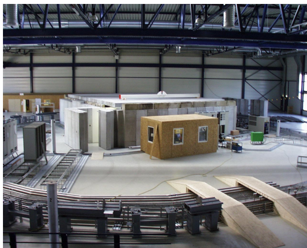
Figure 1: Status of the inside of the building as of March 99, showing the assembled girders, cooling pipes and cable trays. Furthermore the shielding around the microtron and the provisional control room for the commissioning of the injector can be observed.
