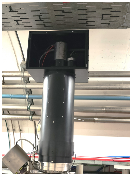
Figure 1: Current design of the OTR-PMT monitor installed in TT20 transfer line in SPS.
