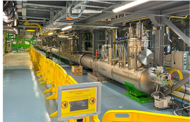
Figure 2: SQXL cryogenic line in the HL-LHC IT String.
