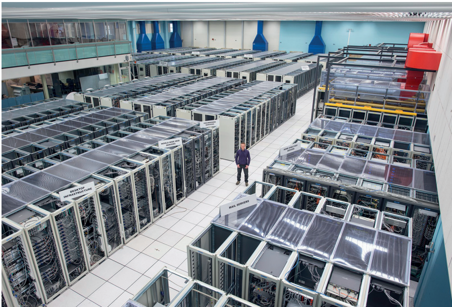
Figure 11.2 CERN's Computing Centre
