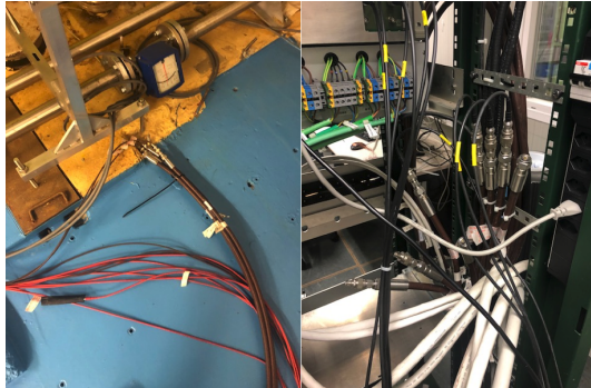
Figure 5: Cable connections in the tunnel.
