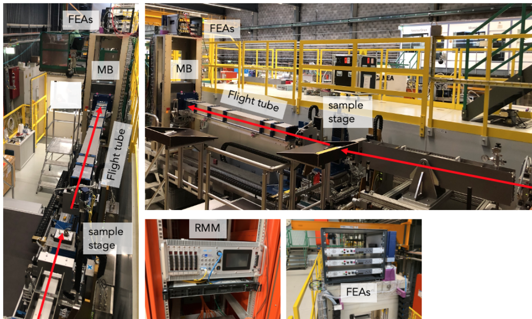
Figure 4. Pictures of the installation at Amor showing the neutron path at the reflectometer in red.
