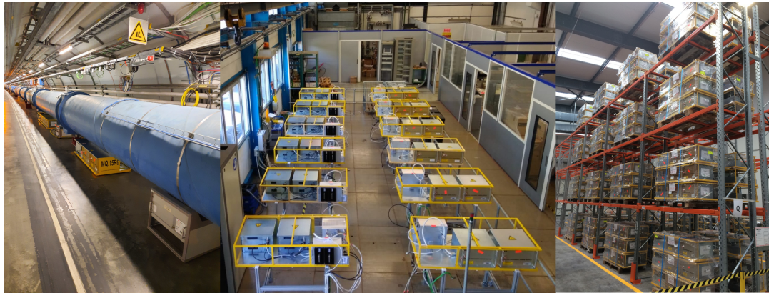
Figure 14. Quench Protection Racks for the LHC Main Quadrupole Magnets in position in the tunnel (left), during the upgrade at the Laboratory (center) and at temporary storage (right).
