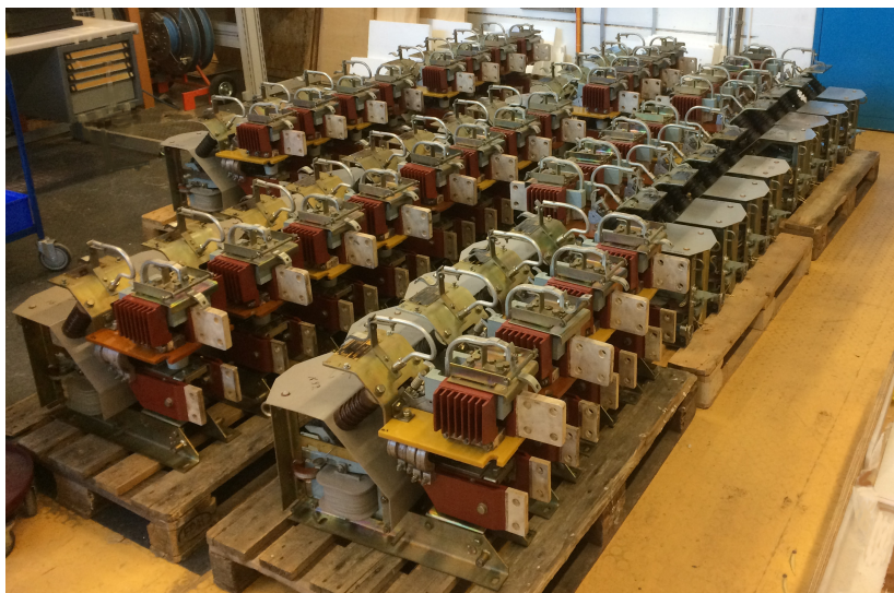
Figure 15. Switches of the 13 kA energy extraction systems in the laboratory.
