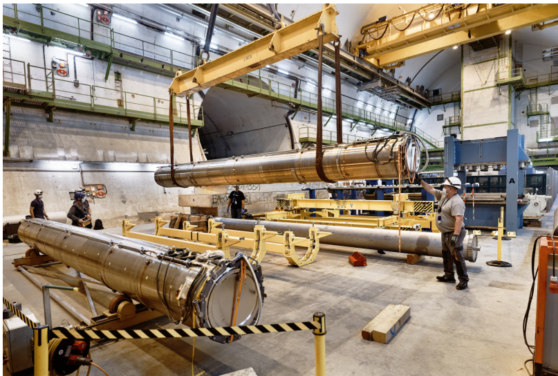
Figure 19. Photo of the two LHC spare dump blocks being equipped in the underground cavern at Point 6 in order to become the new operational dumps. In the figure one could see the dump blocks being inserted in the new cradle as well as the new dump block upstream Ti-Grade 5 window (CERN-PHOTO-202009-112).
