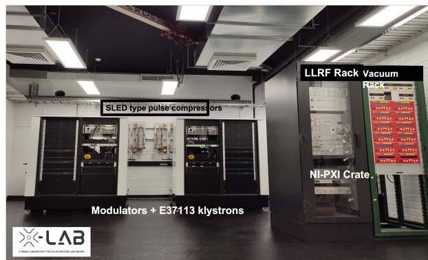
Figure 1: Layout of the new X-LAB and the configuration of the Mel-BOX test stands.
