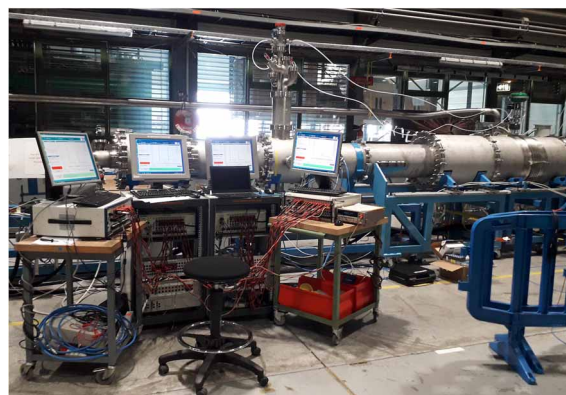
Figure 4: Four DMM Hybrid racks used at the same time during tests of a Superconducting-Link.
