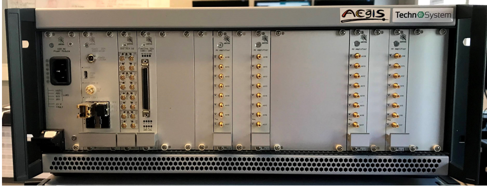
Fig. 1: Photograph of one of three fully equipped Sinara electronics crates of the AEGIS trap control system, including (from left to right) power module, Kasli carrier, digital I/O units, Fastino DAC, and four high-voltage amplifier boards.
