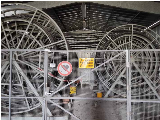
Figure 2: KFA14 (left) and KFA10,20 (right) PFL cable drums in the B305 cable shelter.
