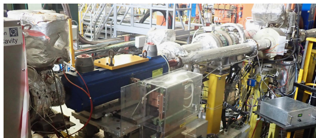
Figure 1: Photograph of the septum magnet SMH40 (blue device). Beam direction from left to right.
