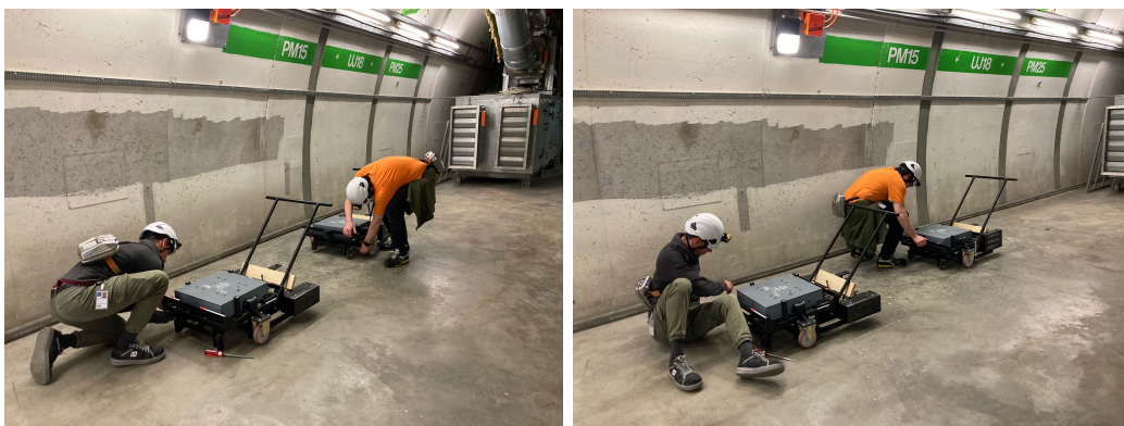
Figure 2.15: Securing the removed walls to the trolley to be transported back on the surface.
