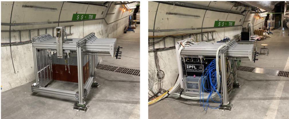
Figure 2.11: Mechanical support of the target system after the installation (left) and fully loaded with wall boxes and SciFi planes (right) [61].
