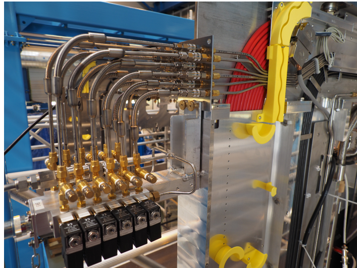
Gas multiplexer for dew point measurements of the exhaust from the coldboxes
