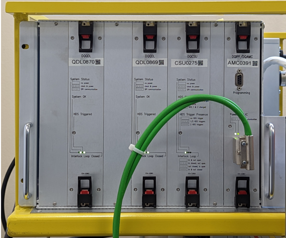
Figure 11. The photo of a quench detection unit installed in the test facility.
