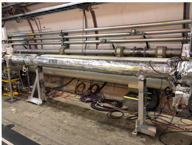
Fig. 3 Conditions inside the LHC tunnel at the proposed location. Good accessibility and space availability allow for easy installation of the crystal assembly
