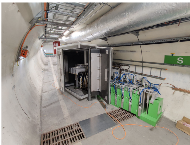
Figure 53. Global view of the detector in TI18 after the installation of the neutron shield.
