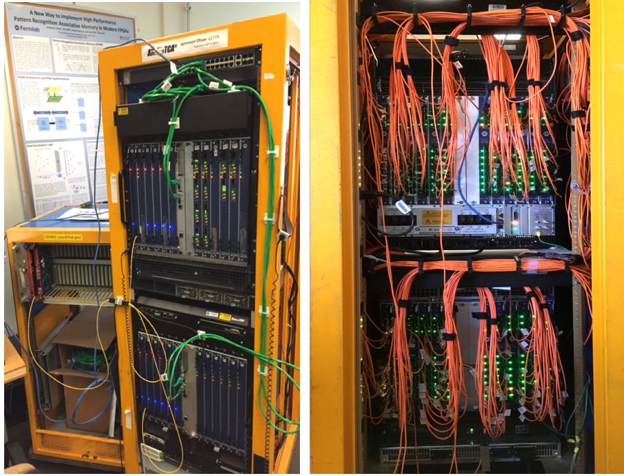
Figure 9: Demonstrator hardware rack. The Data Source boards are in the lower ATCA shelf and the PRBs are in the upper shelf. The rear view of the rack (right) shows 120 QSFP+ optical cables connecting the two shelves.
