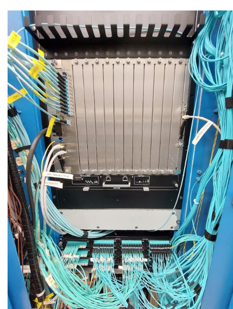
Figure 4: The new MUCTPI installed in the ATLAS service cavern. All of the input fibers from the muon sector logic boards (L1Muon SL) and the output fibers to L1Topo, CTP and the DAQ system are shown.
