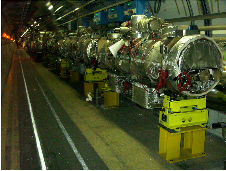
Fig. 1.3 Four MKI kicker magnets in the LHC tunnel.
