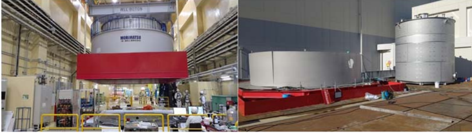
Figure 90. The JSNS 2 detector during the installation (left) and the construction status of the new far detector of the JSNS 2 -II (right).
