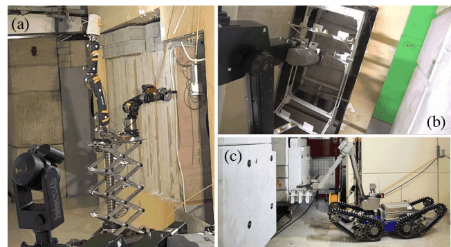
FIG. 9. Three of the main tasks carried out by robots: (a) CERNBot2.0 with double arm configuration cutting cables; (b) Teodor installing the shelf structure on the n_TOF's spallation original target pool; (c) Telex robot installing an intermediate support with six sample containers in the NEAR irradiation station (CERN-PHOTO-202107-085-7) [39].
