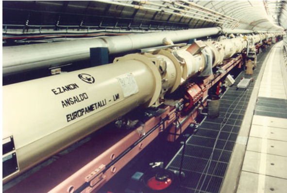
Fig. 6.30 View of the two independent storage rings for electron and proton acceleration in HERA. The super conducting proton lattice is placed on top of the conventional electron ring
