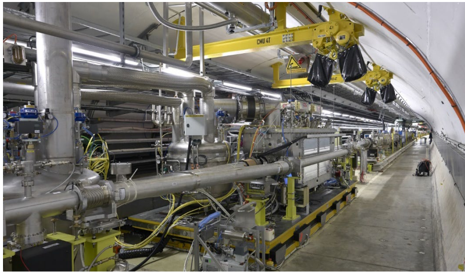
Figure 2: The completed SRF SPS test stand, seen from the direction of the beam. The transfer table is in experimental position; the articulated Y-shaped chamber and cryogenic Service Box with jumper to the DQW cryomodule prototype are clearly visible, while the RF passive equipment is hidden behind the cryomodule.
