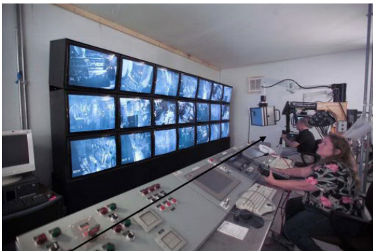
FIGURE 2. The SNS robot control room. It can be noticed the complexity of the control room equipment [34].
