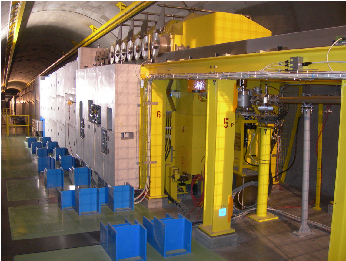
Figure 4.4: Photo of the CNGS target cavern with the target station in the forefront. The slope of the tunnel required to point to Grand Sasso is visible.
