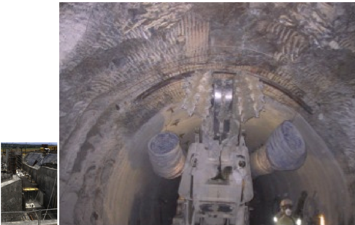
Figure 6.8: Cut-and-Cover excavation technique at LINAC4 (left) and the road header machine (right)
