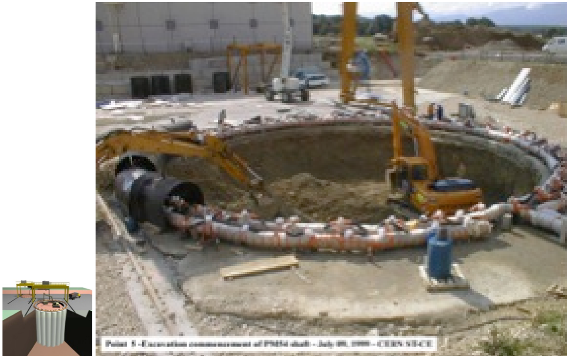
Figure 6.9: ↗Cut-and-Cover↖ excavation technique at LINAC4 (left) and the road header machine (right)
