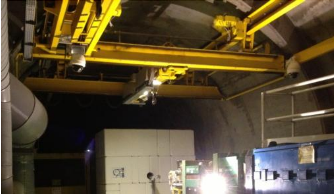
Figure 6.33: Photo showing the CNGS remotely operated overhead crane after the onboard camera and lighting upgrade.
