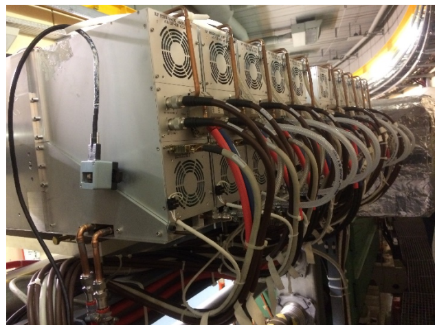
Figure 4: Solid State Amplifiers to drive the wideband cavities.
