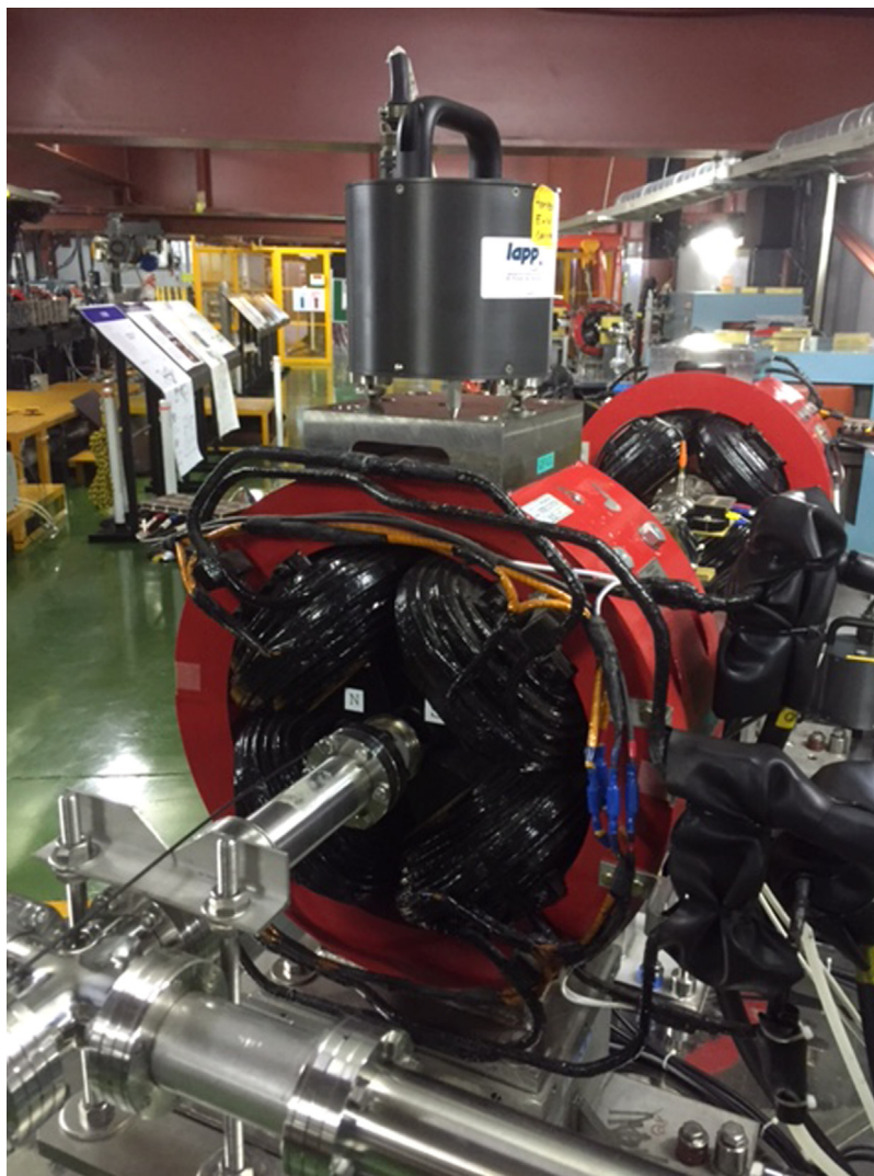
Fig. 3. Photograph of the seismometer mounted on quadrupole QF4X.
