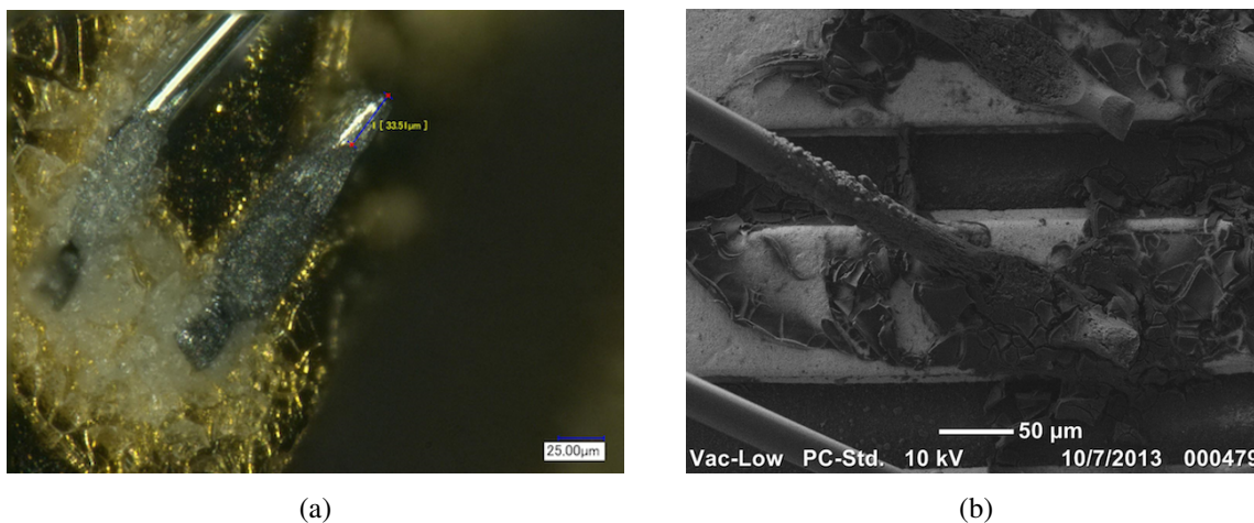
Figure 46. (a) White residue of corrosion on staves as observed under a microscope. (b) A Scanning Electron Microscopy (SEM) image of corroded wires and the corrosion residue at the foot of the bond.
