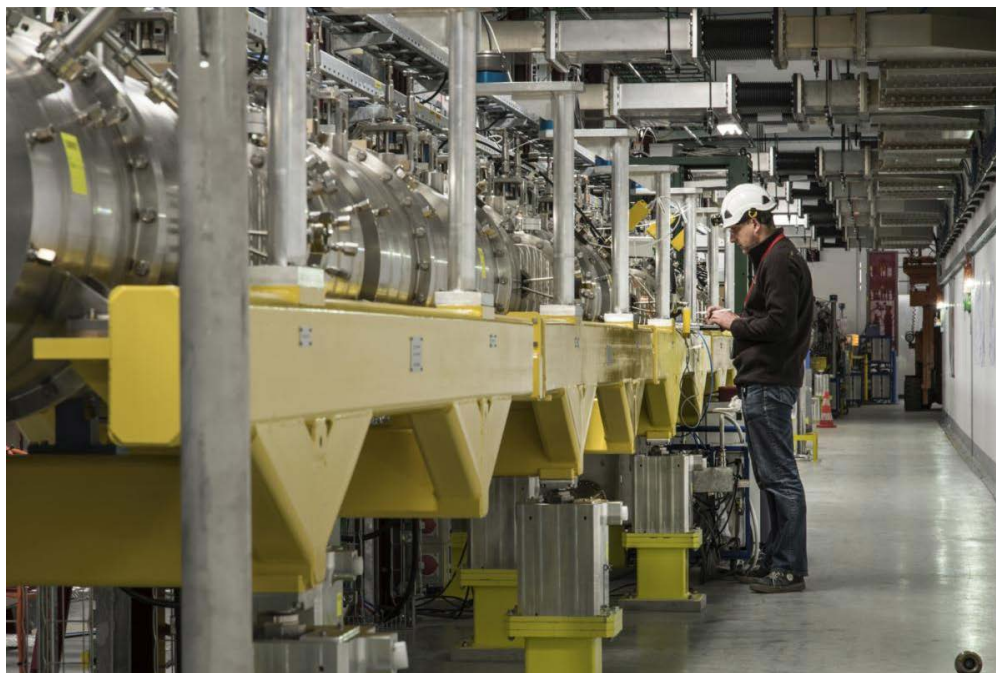
Installation of the CCDTL structures of LINAC4, built and assembled in Russia (Image: CERN CDS)
