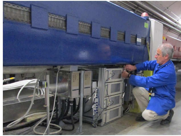
Figure 15: Two wideband 5 - 1000 MHz amplifiers installed in the SPS tunnel as part of the upgrade to use 1 GHz bandwidth vertical kicker striplines. Two more additional amplifiers will be installed in 2016 to power the second stripline.
