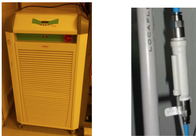
Figure 5: The chiller (left picture) and the flow switch (right picture).
