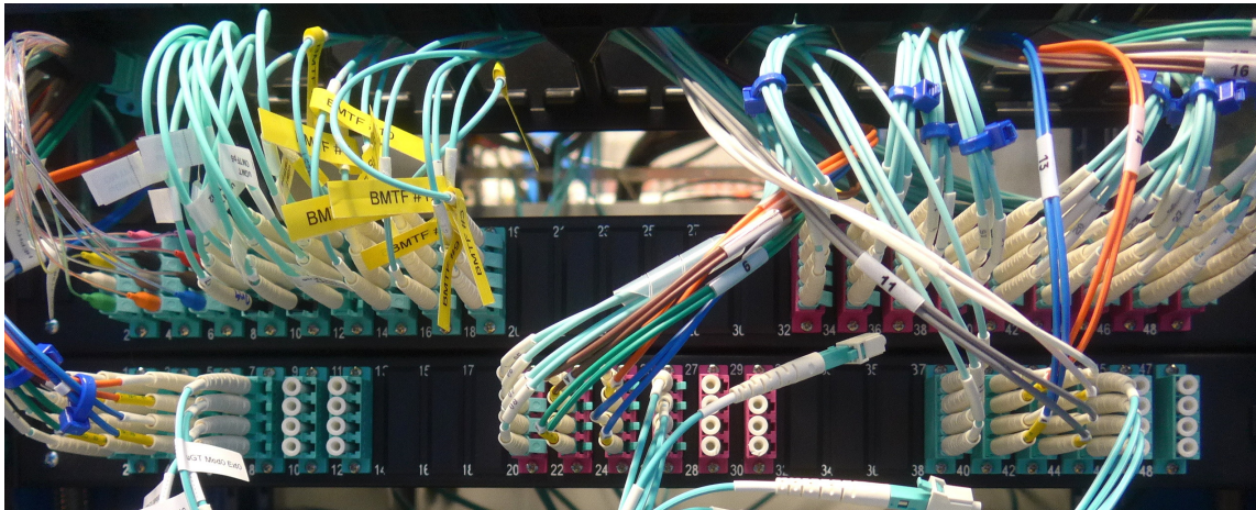
Figure 3. Optical patch panels guarantee the connections between the different subsystems.
