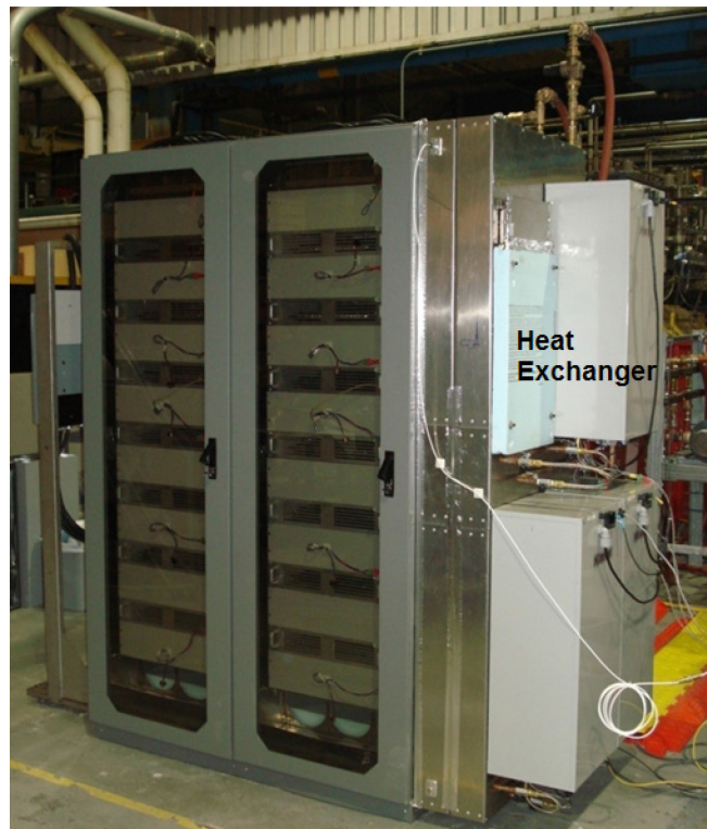
Fig. 8: NSLS-II sealed racks (equipment enclosures)
