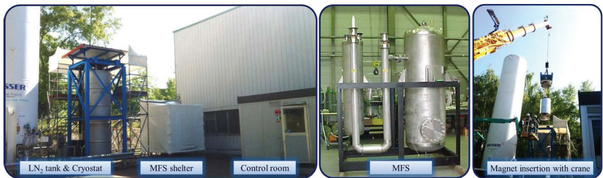
a) b) c) Fig. 1. a) Global view of the Nitrogen Test Facility at CERN; b) view of the Magnet Flushing Station; c) view of the FRESCA2 insertion.
