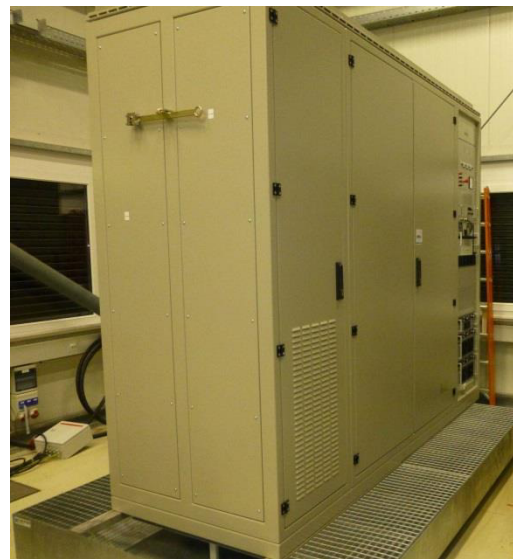
Figure 7: Klystron modulator installed in place.
