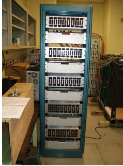
Figure 16. Photograph of the low voltage power rack containing five pairs of low voltage power supplies and distribution boxes.
