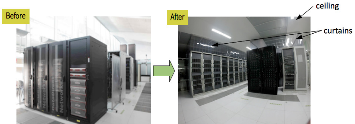
Figure 4. PIC main computing room before (left) and after (right) completion of hot/cold air separation and confinement.
