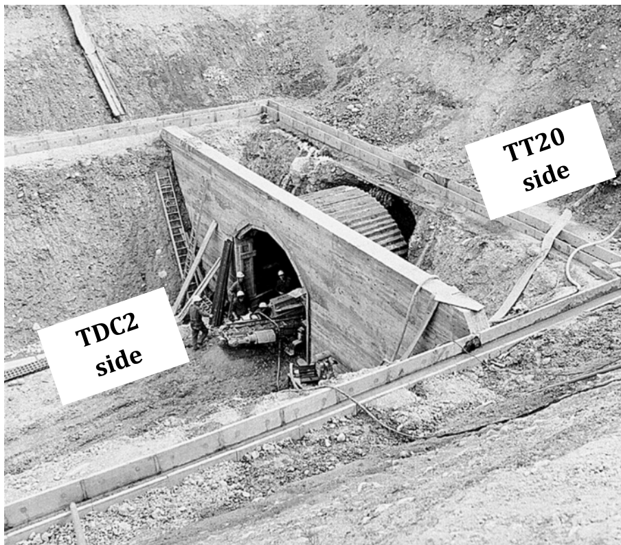
Figure 4: Photo from May1972 showing the start of tunnelling for TT20 line going down to SPS.
