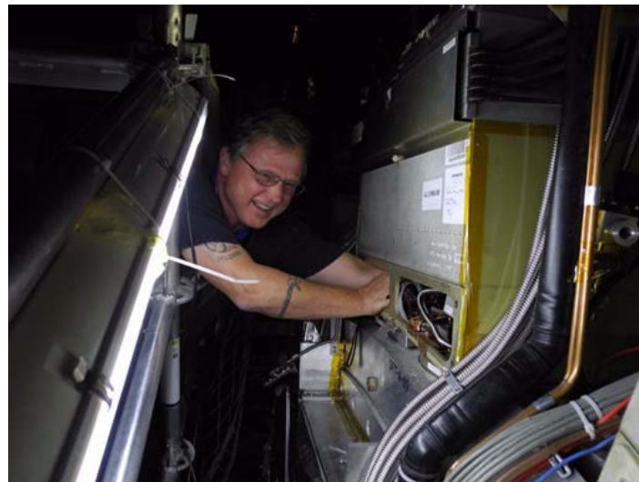
Plugging warm cables into new backplane
