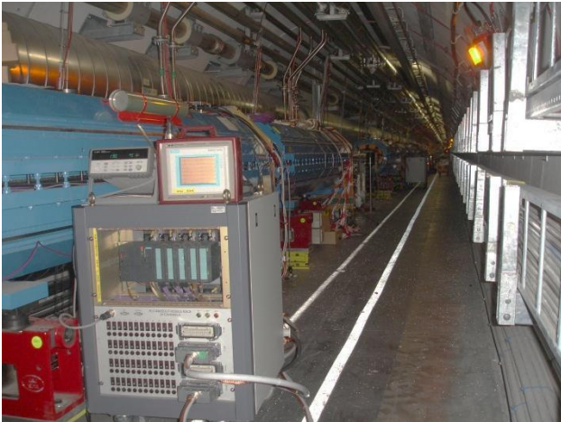
Figure 2: Bake-out mobile cabinet in the LHC Tunnel
