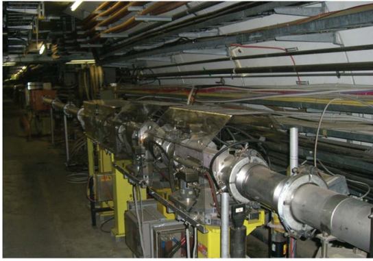
Figure 10: SPS BBLRs no. 1 and 2 (4 boxes) installed in SPS Straight Section 5.
