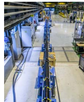
Fig 1. The 20-metre long electrical transmission line containing the two 20 kA MgB 2 cables.
