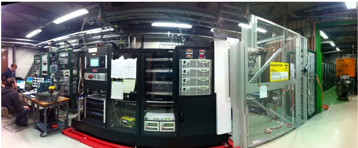
Figure 1: A photograph of the Xbox-1 test stand. The control and low-level rf systems are to the left, the modulator is in the middle and the high-power rf network is to the right. The test accelerating structure is located in the former CTF2 accelerator bunker located in the floor below.
