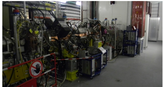
Figure 1: The Linac4 3 MeV section (from right: ion source, RFQ, chopper line) installed in the tunnel.
